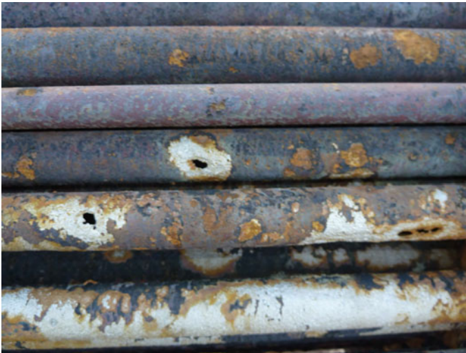
Fig. 9 Zone tube bundle corrosion damage (Zone 3)
